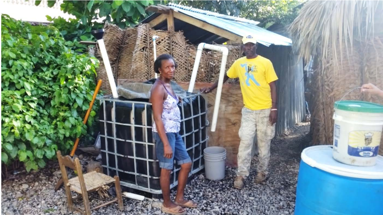
Bibine and Charles standing by the bio-digester close to the kitchen
